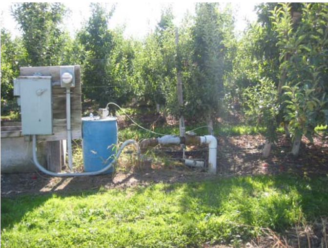
LeFore – Fifty pumping station
