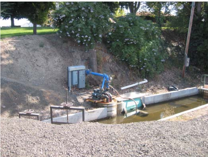
Schmidt & Sons Nursery – Diversion pump
