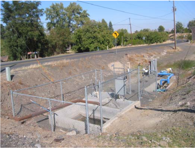
Eastside Diversion – Head box
